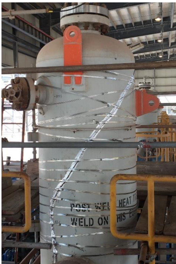
Figure 7. FBG sensor cable mounted to pump discharge accumulator.
